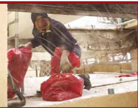
Removing debris of contaminated sprayed coatings at Newcastle University (picture taken from behind protective screen).
