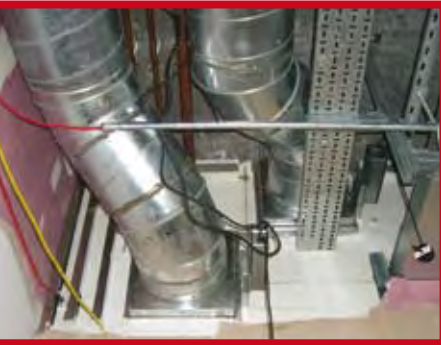
Fire stopping around services penetrations in walls.
