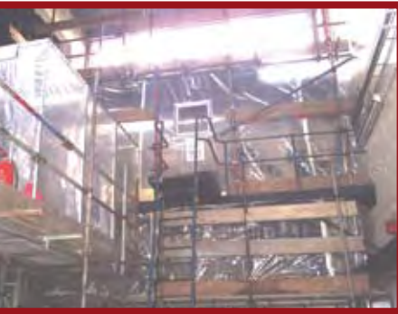
In 2007 Chirmarn completed one of the largest asbestos removal projects in the UK prior to the demolition of Newcastle brewery.
